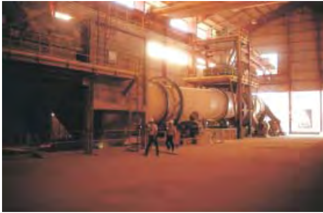
Figure Togo 12. Togo Beneficiation Plant, Rotary Dryer
