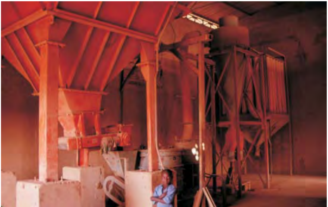
Figure Niger 9. Grinding Mill, Cyclone and Bagging Station, Tahoua
